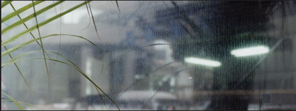
Severe moisture attack beyond the “point of no return”
