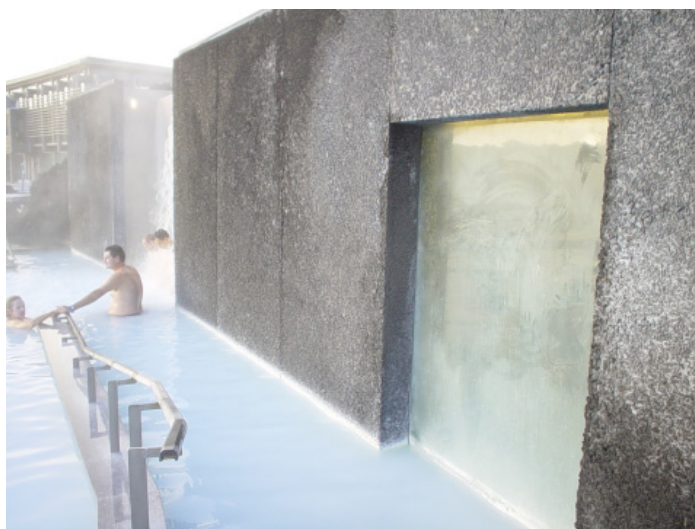
Heavy silica contamination on a glass door at the Bláa Lónið resort prior to ClearShield renovation and protection
