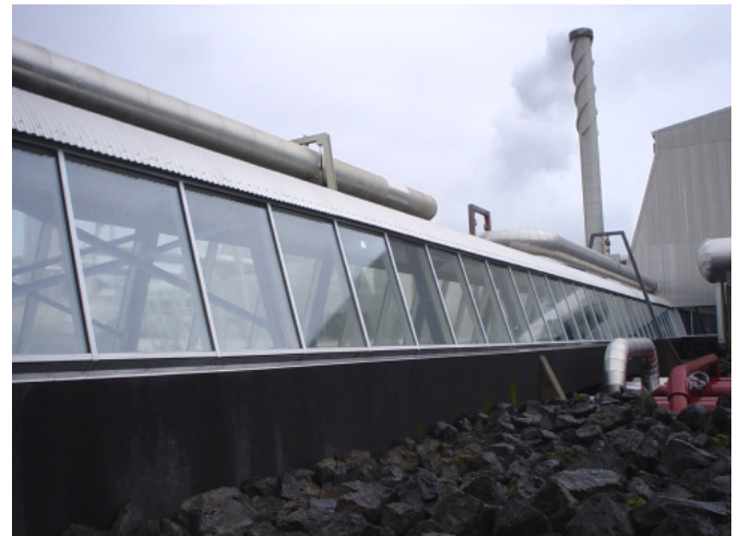
Today, glass at the power plant looks newer for longer and is always easier to clean thanks to ClearShield
