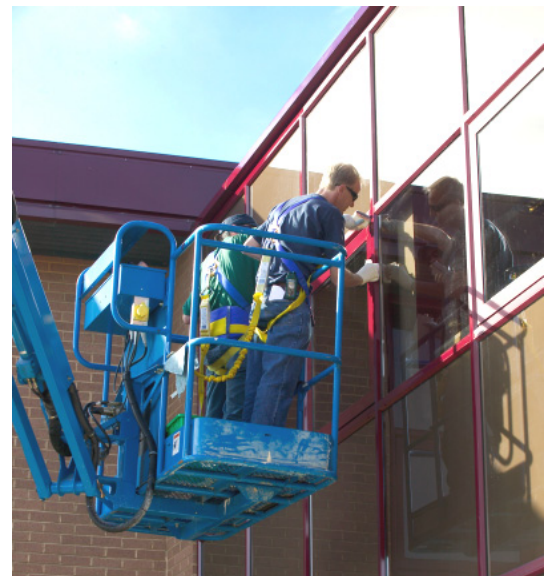
The specialist Ritecoat team utilising a cherry picker to access higher areas
